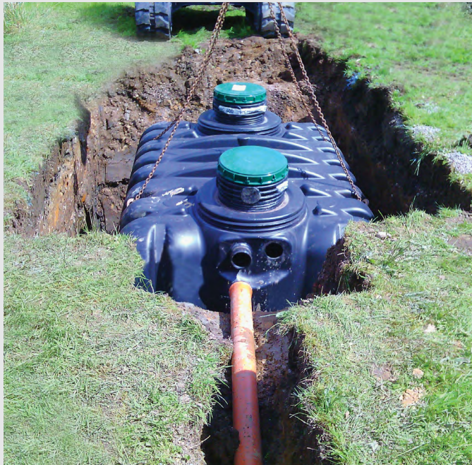
Tricel Vento installed.
